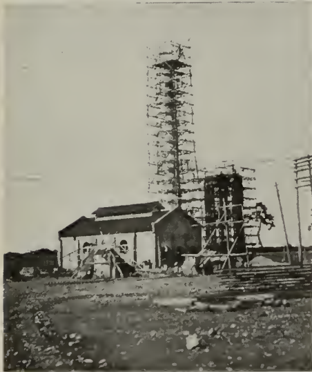
Power Plant at Hanazana Mill. Reinforced concrete chimney built entirely by man power, no machinery being used. Staging was built with bamboo and straw rope, no nails used
