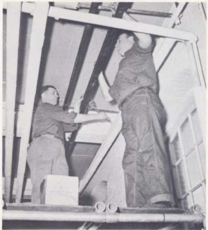
The new heating pipes being installed by John Farrar, left, and Joseph A. LeFrancis, right, will be concealed by a modern ceiling. Note that the under surface of the floor above has been sheathed with fireproof board. These men are from Department 668
