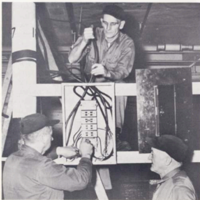
While the work is in progress, a number of temporary installations have to be made. On the right George Rae, a supervisor in Department 470, watches as electricians Joseph Stefans, left, and Robert Blackburn, center, wire a temporary lighting cabinet
