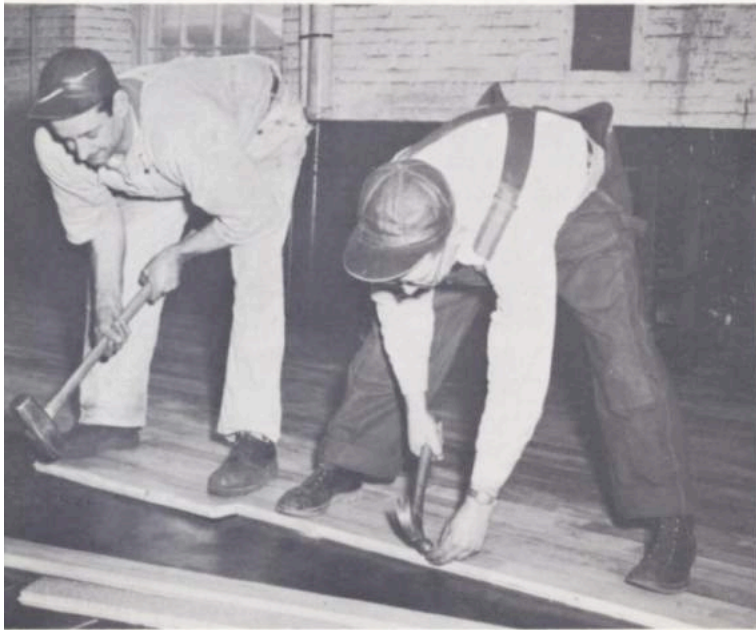
The old flooring, worn by years of industrial use, has been replaced by gleaming new maple. Henry Lavine, left, and Charles Bouvier, right, two carpenters from Department 670, make sure that the new floorboards fit tightly
