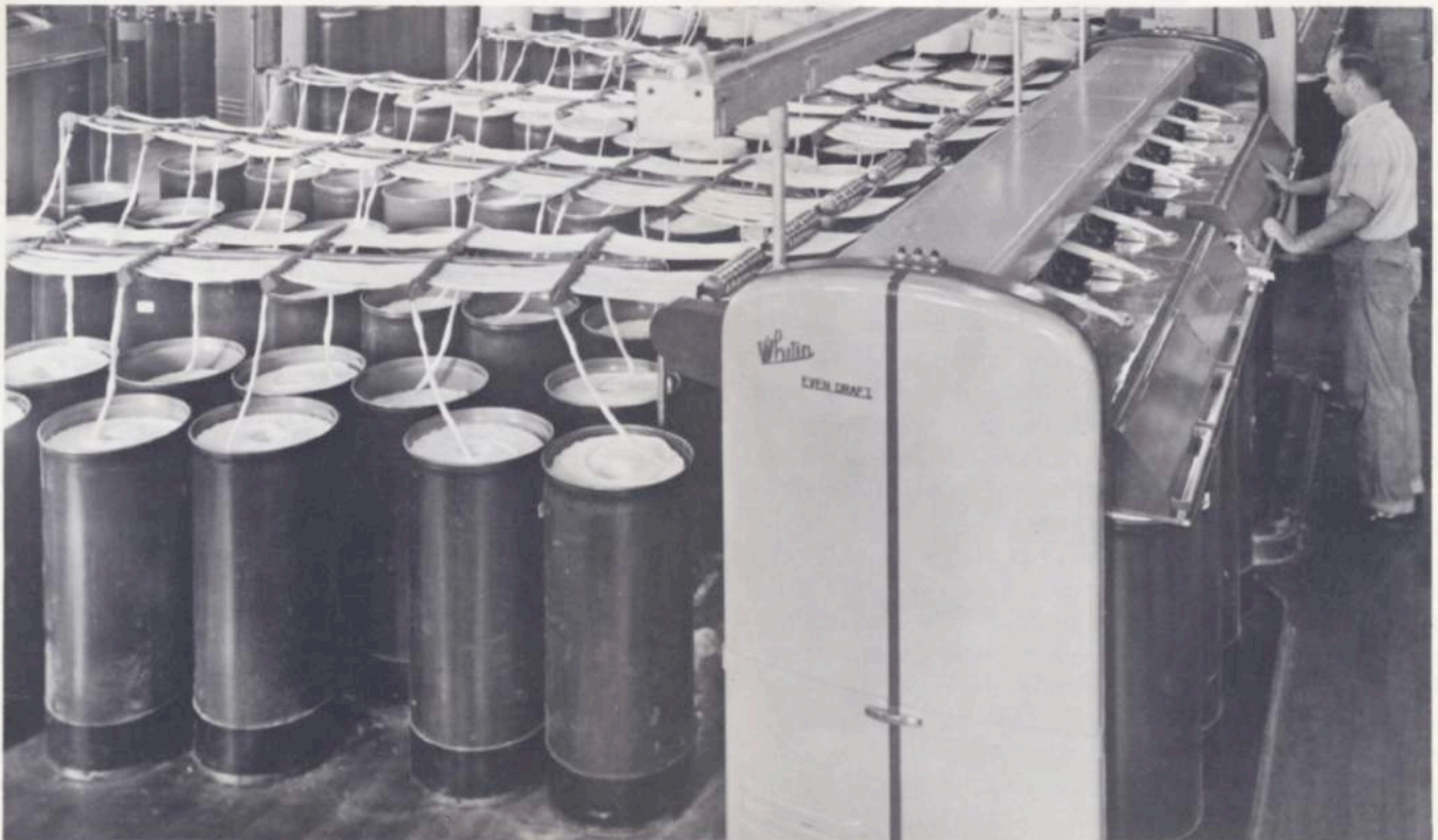
This is an installation of Whittin Even-Draft Drawing Frames at Henderson Cotton Mills, Henderson, North Carolina. A number of slivers from the cans at the left enter the machine to be drawn and combined into a single sliver at each delivery. The resulting uniform sliver is coiled in the cans shown at the right. Thomas Boroday, a serviceman, checks the operation of the machines
