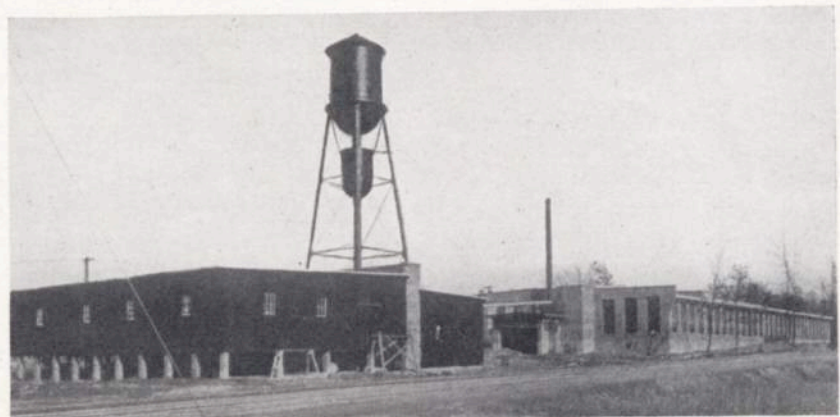
A View of the Carlton Yarn Mill, Cherryville, N. C. Built in 121 Working Days. A Record in Mill Construction
