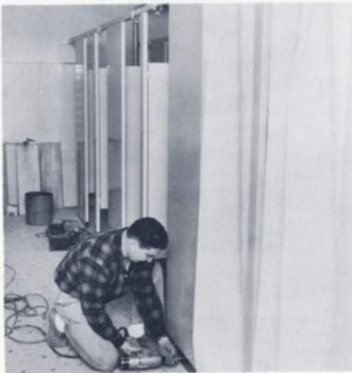
In a new yellow ceramic tiled shower room for women, 15 individual shower compartments have been installed
