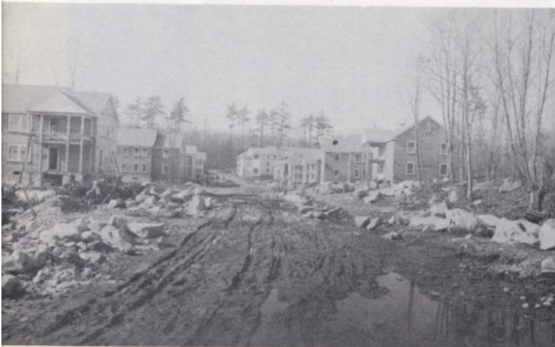
During this decade, when the Plummers section was built, a great deal was spent on highway improvement. When this photograph was taken on March 11, 1921, the houses on Leland Road were only partially completed
